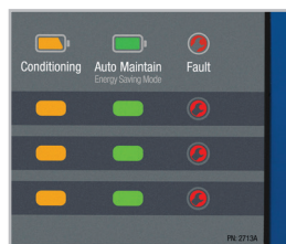
Battery fault detection LEDs
